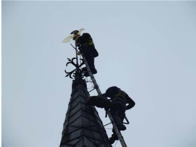
Steeplejacks from Dawsons reattaching the weathercock to the spire of St James after repair and re-gilding
